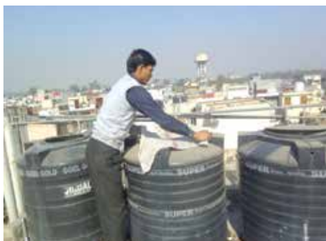
Overhead water tanks
